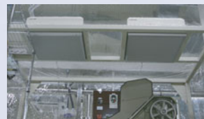
Two HEPA-filter units fitted in the booth
